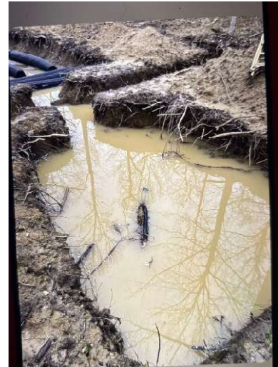
Flooded Septic Bed
